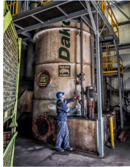
A core scrubber removes spent gas from the core making process before the air is discharged.
