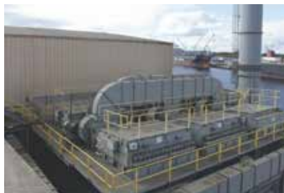
State-of-the-Art Pollution Control
